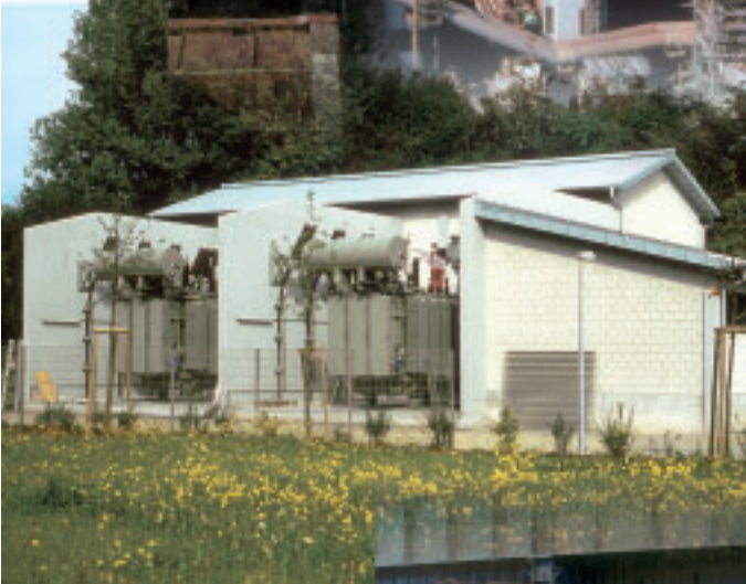
Application Public power supply system
